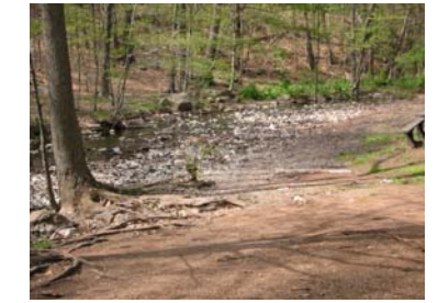
Figure 20 ~ Tulip Spring: Severe erosion and compaction threatens trees. Bank configuration is compromised and utilities are exposed.
