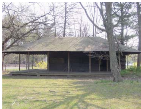
Figure 80 ~ Abandoned building at the Oakdale picnic area.
