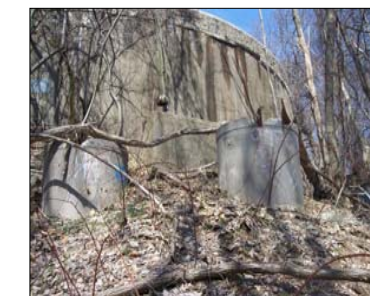
Figure 41 – Low side of NJ American Water Holding Tank and access towers.
