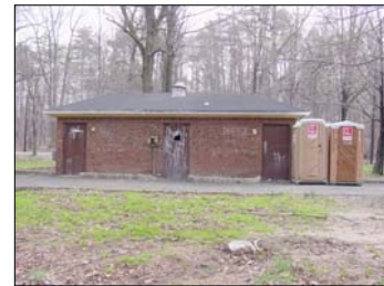
Figure 59 – Non-functioning restroom building with port-a-potties servicing area
