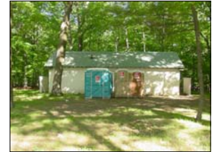
Figure 76 – Turtle Back Picnic Area restroom facility provided by porta-johns as the building does not function.
