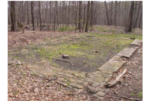
Figure 90 ~ Remnant of picnic shelter foundation at Shady Nook picnic area.
